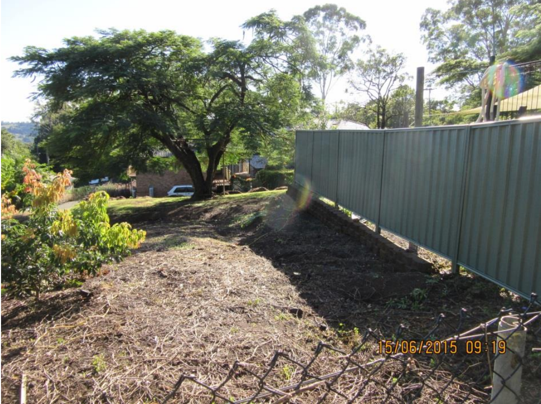
Start of swale drain system No. 1 Gladioli Avenue adjacent to shared boundary
